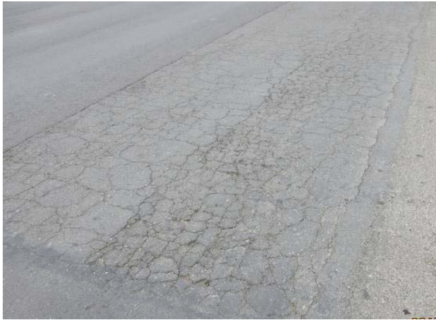
▲沿線路面龜裂不平整
